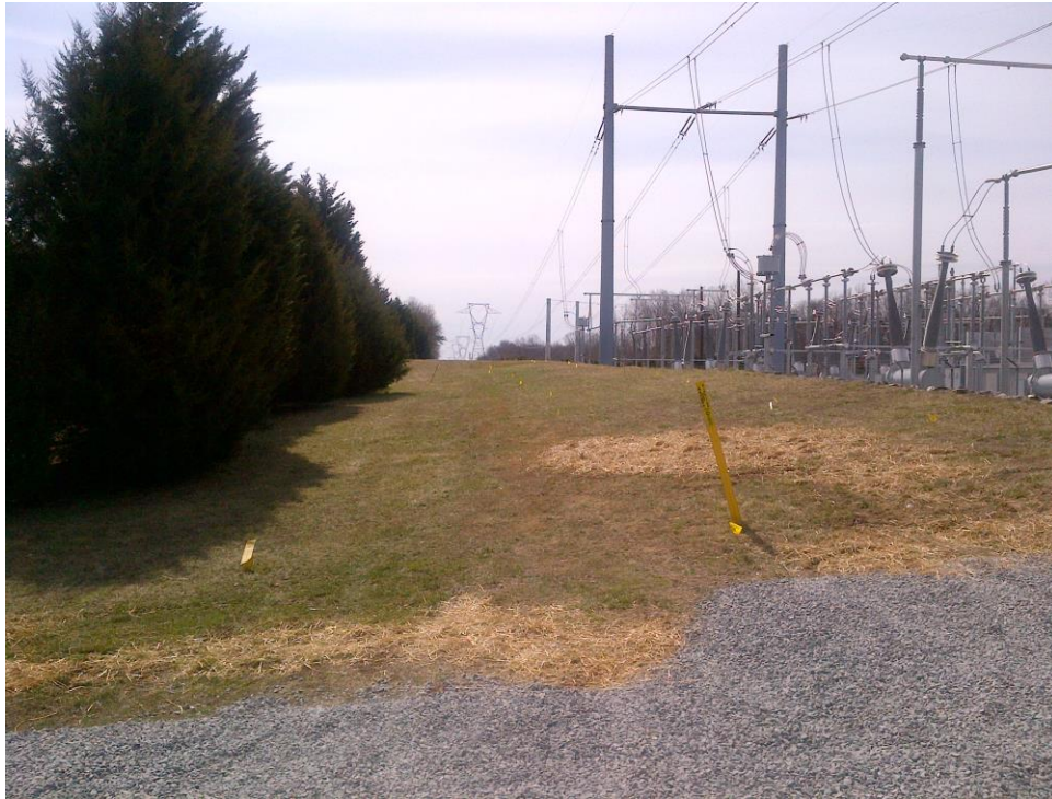
Power Line Structures-North
