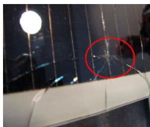
Fig. 2. PV module with fractured glass (impact, edge breakage).
