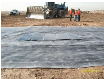
Fig. 5. Aljon model 91K compactor used to crush PV modules in a Municipal Solid Waste Landfill in the State of Arizona, USA.
